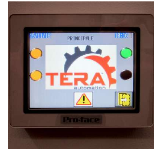
PLC + HMI touch screen
